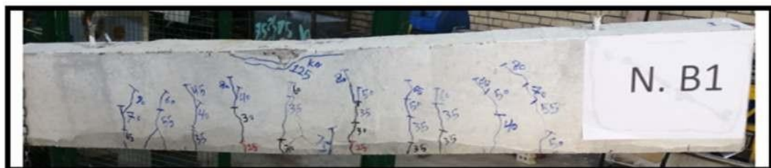
Plate 2. Cracks Pattern of CB.
