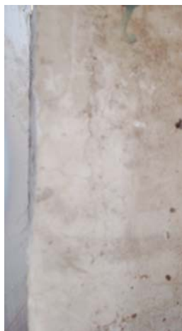
A- Column specimen C 4 after exposure to 500 °C and cooled suddenly
