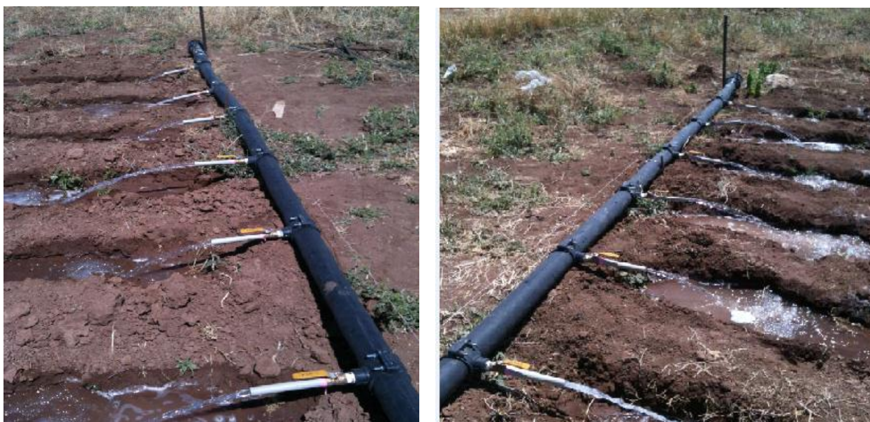
Figure (4): main line pipes on both sides
