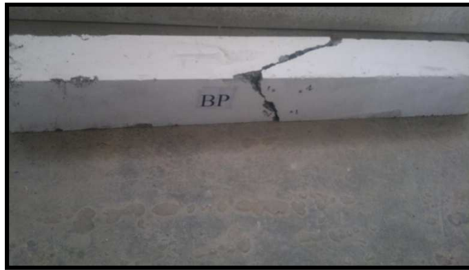
Figure (13), Failure Mode of High Strength SCC Beam (Bp)
