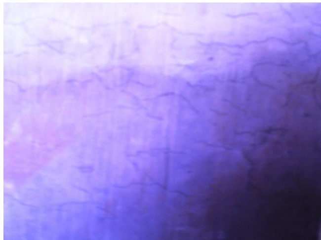
Plate (7) Thermal Cracking in panels without PPF
