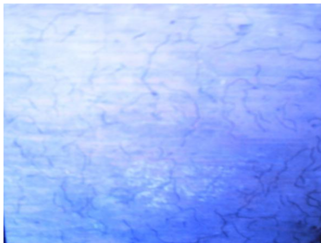
Plate (8) Thermal cracking in panels with (0.4%)PPF
