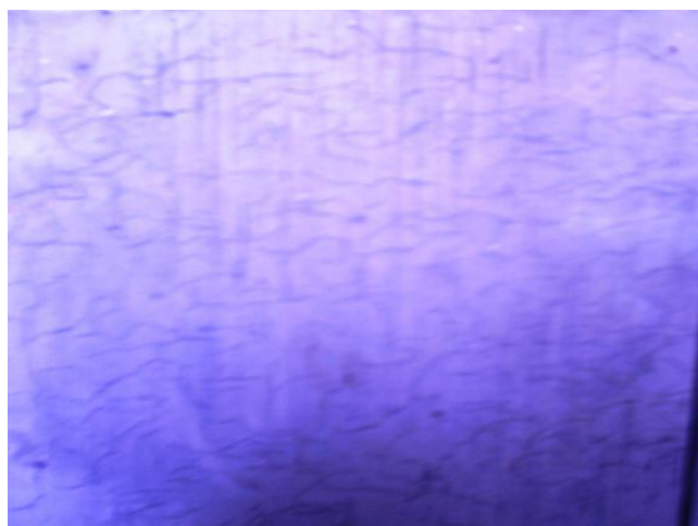
Plate (9) Thermal cracking in panels with(0.8%) PPF
