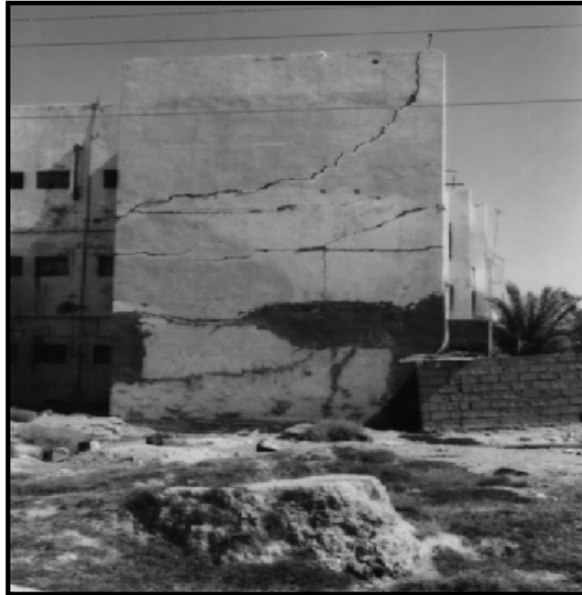
Figure (1) Collapse of a building in Al-Ramadi City, (From Tawfeeq, 2009).
