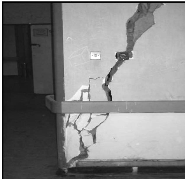
Figure (2) Cracks of Walls in Dijla Hospital in Tikrit City,(From Tawfeeq, 2009).
